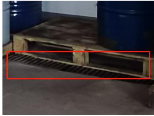
危废暂存间收集边沟
